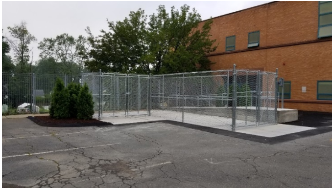
Top to Bottom: Moylan, S.A.N.D and Classical Magnet Schools; Construction Progress Photo
